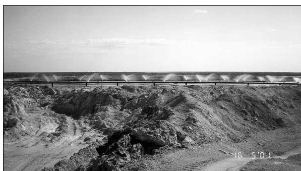
Fig. 5. The excess water evaporation system (sprinkling devices) in the 2nd ash field of the BPP
